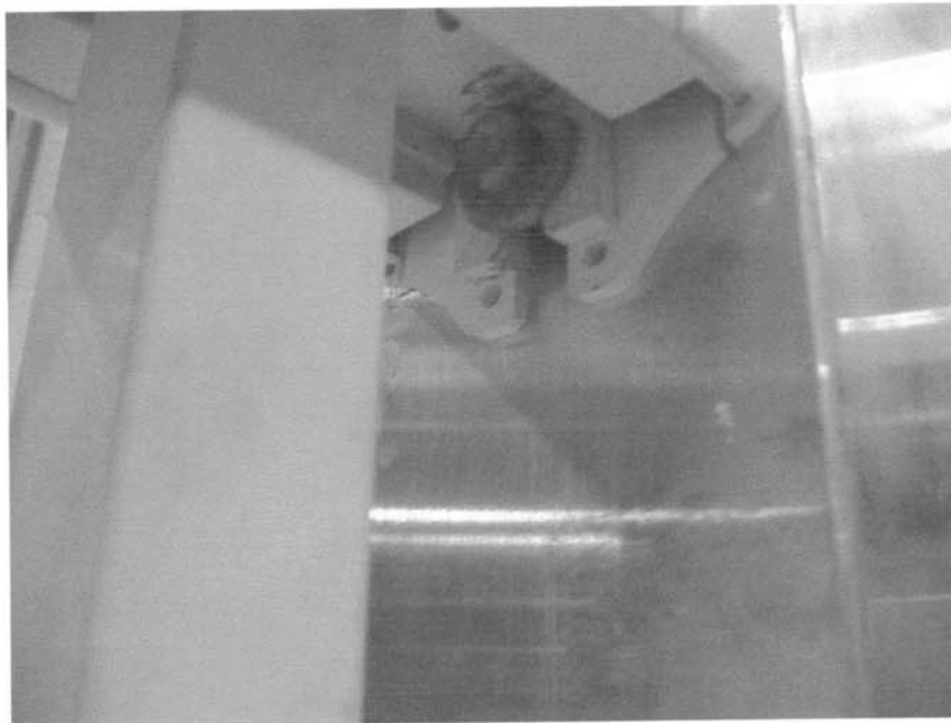
Photo No. 4 Top Rail Bracket Assembly
