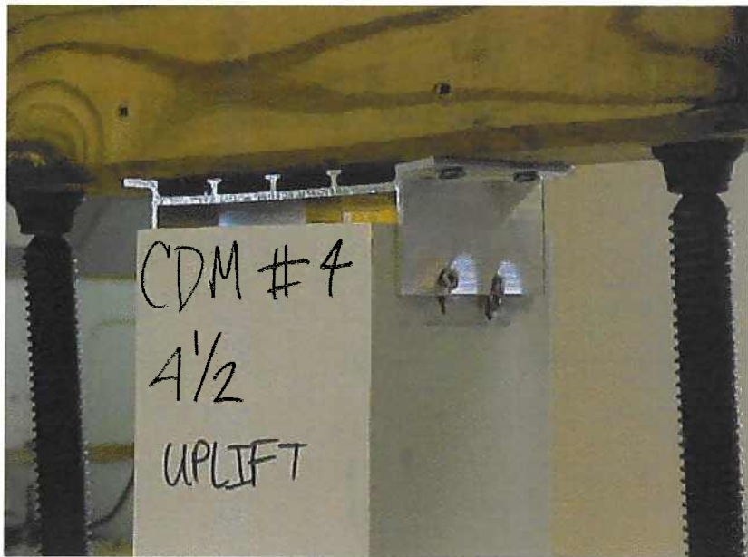
Photo No. 7 4-1/2" by 4-1/2" Porch Post Bracket Failure
